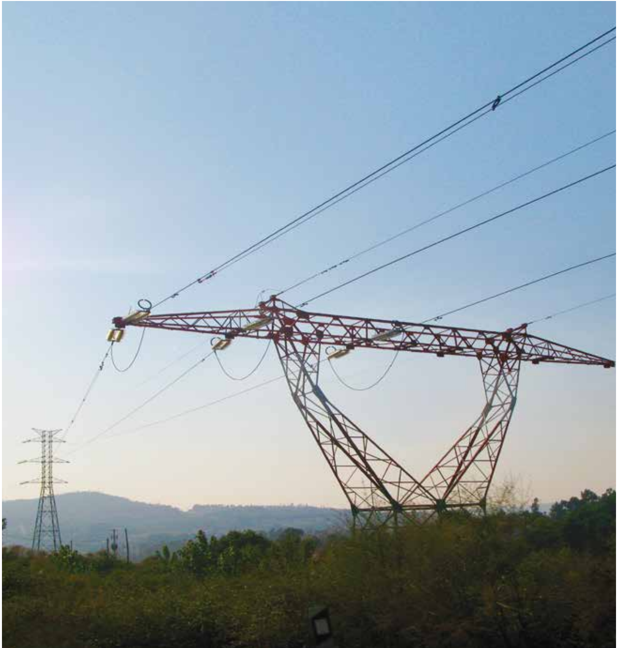
Photograph: High voltage towers / Source: Chile Sustentable.
